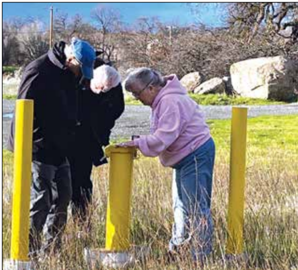
From left, Lincoln City Councilman Bill Lauritsen, Ray Birge and Anne Constantin Birge, members of the grassroots Titan 1-A Missile Site Environmental Contamination and Remediation Committee, were looking at the number of the monitoring well to see what the trichloroethylene (TCE) levels have been over the years.
