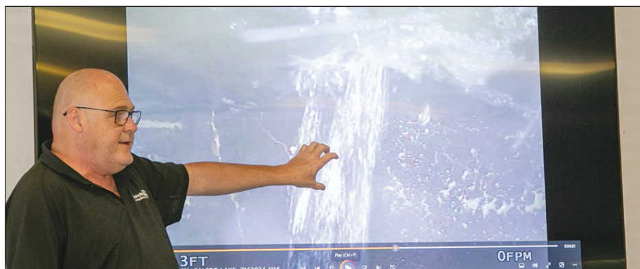
Interim Director of Operations Travis Bohannon points out a leak in a video taken of a crucial pipe that carries raw water from the Cosumnes River to Calero Reservoir. The Rancho Murieta Community Services District board authorized him to make emergency repairs at the July 17 meeting. Photos by Gail Bullen
