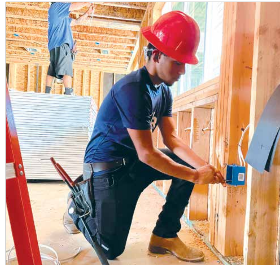
Julian Aguilar works on an electrical installation at a Taylor Morrison home in the Vineyard neighborhood in Sacramento County. Photo courtesy of The Write Stuff Communications
