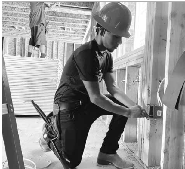
Julian Aguilar works on an electrical installation at a Taylor Morrison home in the Vineyard neighborhood in Sacramento County. Photo courtesy of The Write Stuff Communications
