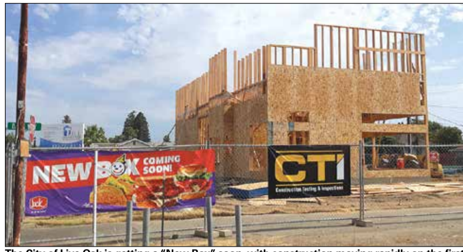
The City of Live Oak is getting a "New Box" soon, with construction moving rapidly on the first drive-thru fast-food restaurant to come to the city, Jack in the Box. Photo by Mickey Mrakuzic
