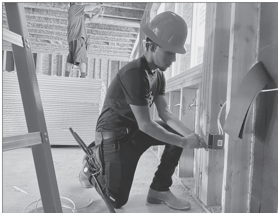
Julian Aguilar works on an electrical installation at a Taylor Morrison home in the Vineyard neighborhood in Sacramento County. Photo courtesy of The Write Stuff Communications
