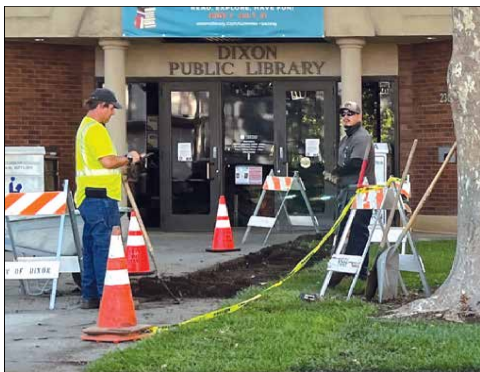
City of Dixon workers broke out a swathe of concrete near the Dixon Library's front doors this past week and replaced it with compressed granite as they ready the ground for the addition of one or two benches to be installed soon. The benches will be courtesy of the Dixon Women's Improvement Club and the Dixon Historical Society. Photo by Debra Dingman
