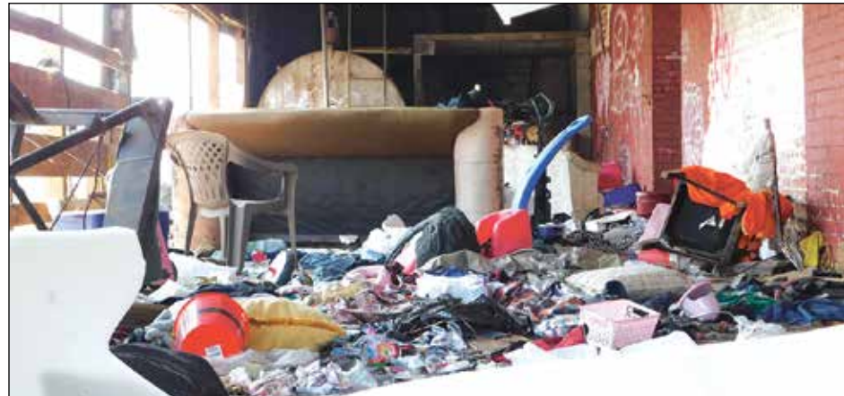
Here is a close up photo of the interior conditions of the building located on the southeast corner of Magnolia and Vermont streets in Gridley. It illustrates the extent of debris and filth that is strewn throughout the structures.
