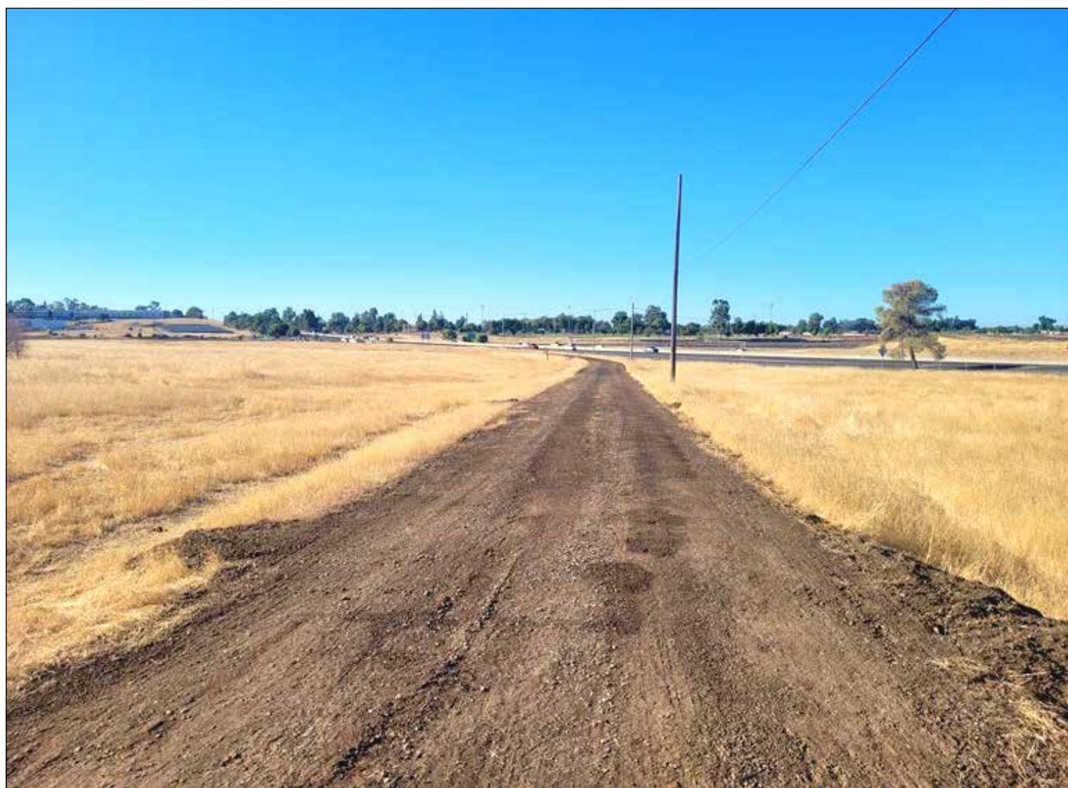
A section of the Brad Freeman trail near Garden Drive in Oroville is prepared for future paving work. Photo courtesy of the Department of Water Resources
