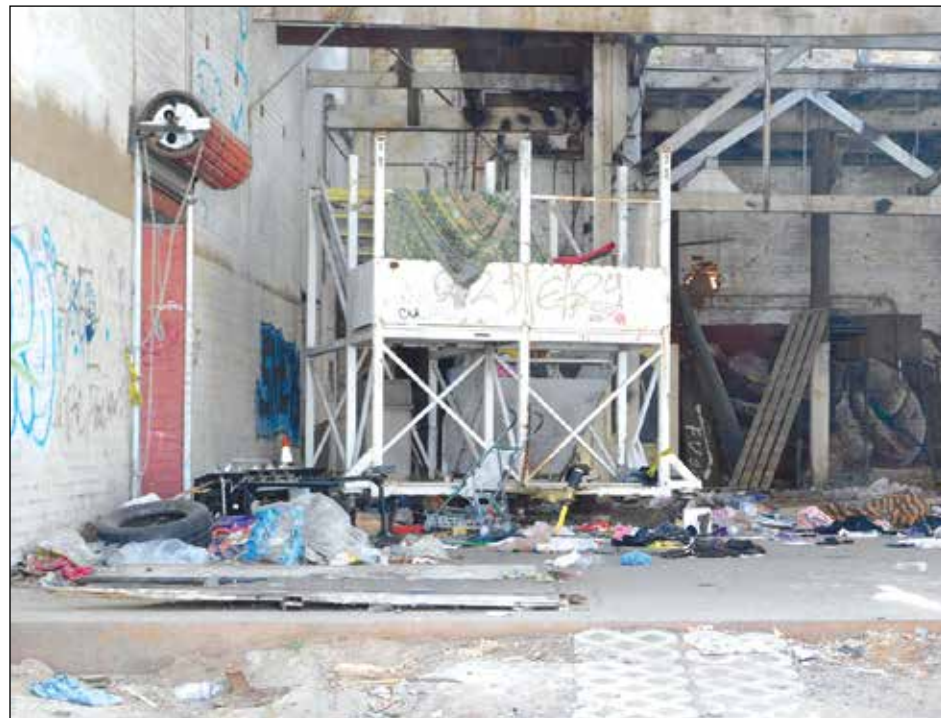
The structures have been a source of serious concern and frustration for Gridley residents and business owners for a long time.
