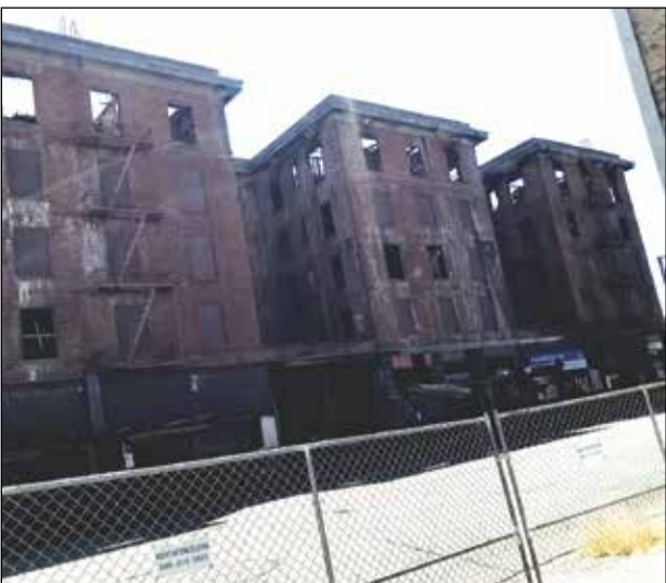
Hotel Marysville is still standing and poses a safety hazard.
