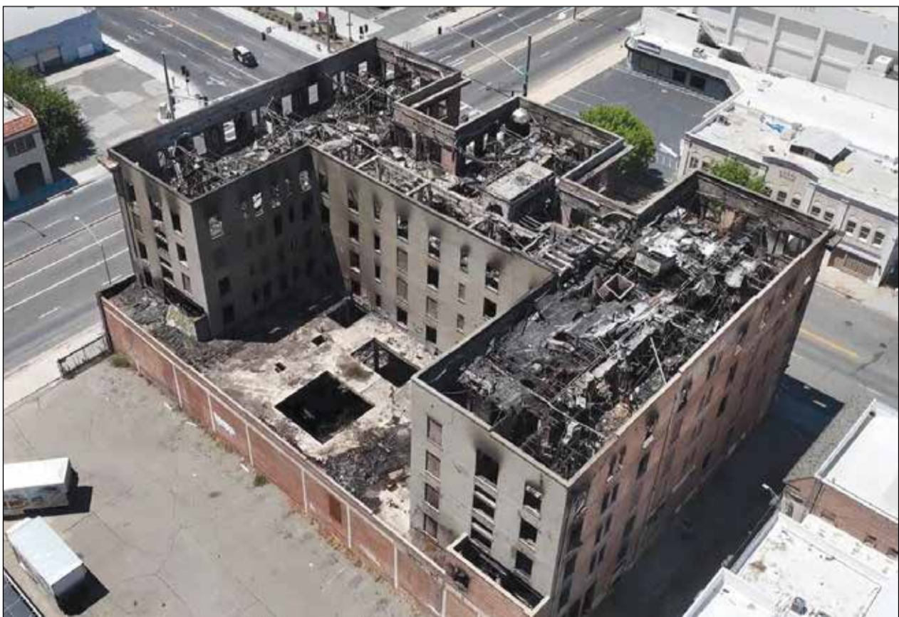
Pictured here is an aerial view of Hotel Marysville's current state. Photo courtesy of the City of Marysville
