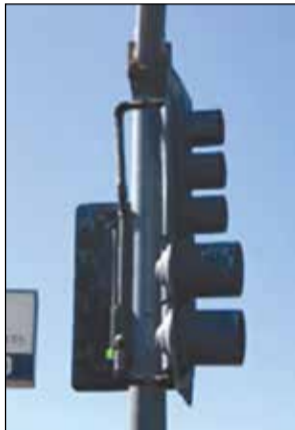
Yuba City has different types of traffic signals, depending on the street location and visibility, and these signals will be upgraded with a new California Local Highway Safety Improvement grant. Photo courtesy of Yuba City
