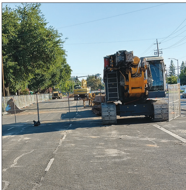
Heavy equipment is on site in the northbound lanes of Franklin ahead of the project's excavation.
