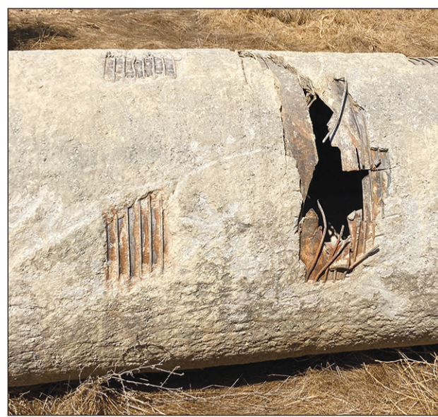
A section of pipe with a huge hole is being replaced in the line that conveys water from the Cosumnes River to Calero Reservoir. Photo courtesy CSD
