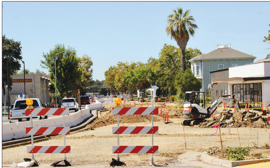
Here is a view of the C Street closure looking west from South Lincoln Way.
