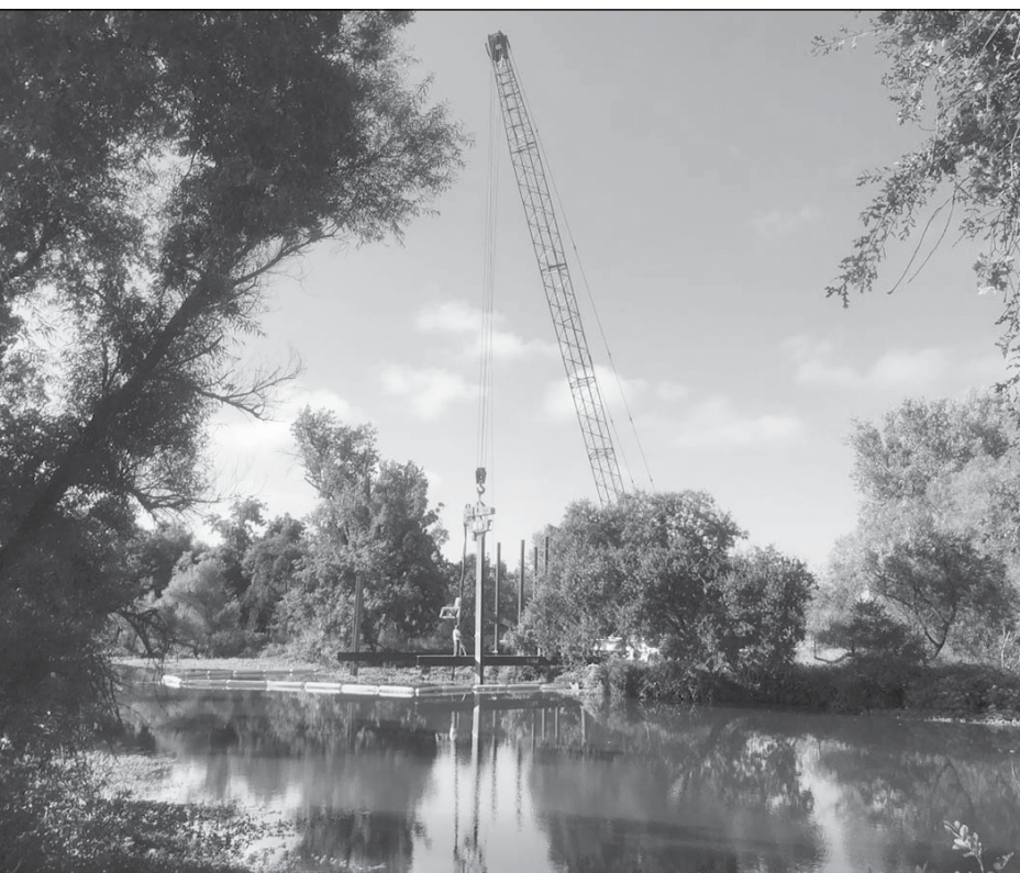
Piles being driven for the new Sutter NWR lift station project. Photo courtesy of Ducks Unlimited
