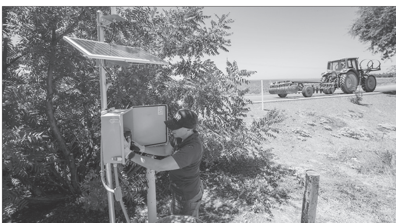
California Department of Water Resources employee Katy Janes, Groundwater hydrogeologist in the Geology and Groundwater Investigations Section of the Division of Regional Assistance North Central Region Office, installs new telemetry equipment in groundwater monitoring wells in Colusa County on July 24. Photo courtesy of California Department of Water Resources
