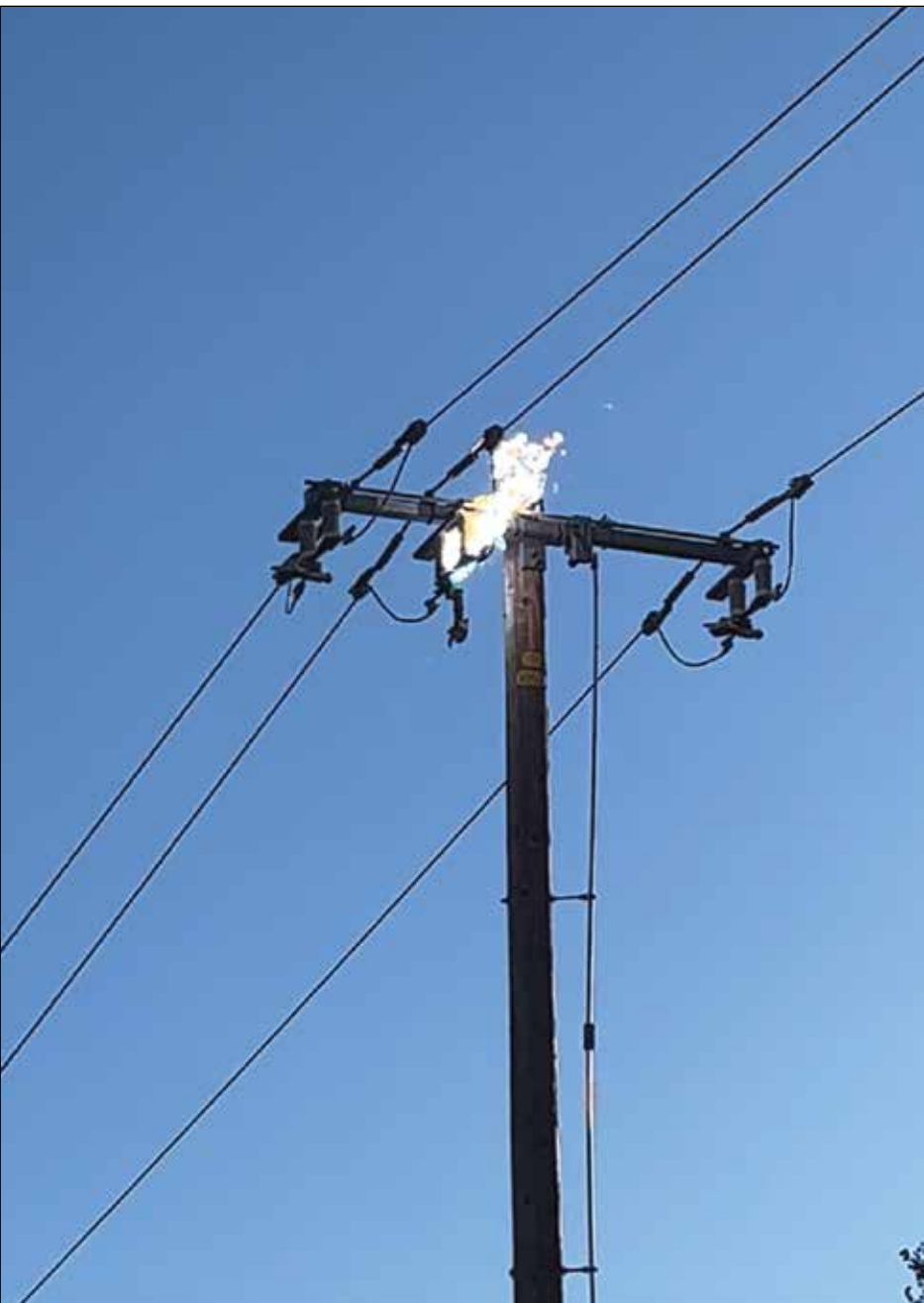
PG&E was dispatched to the scene to extinguish the fire and repair the switch. Photo by Katie Voss
