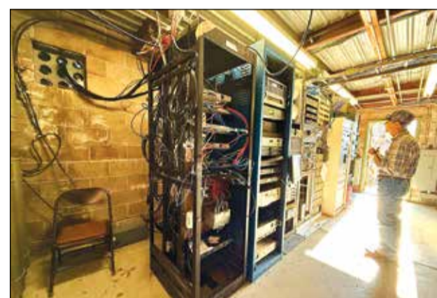
The interior of a community vault is referred to as "spaghetti mess" by Jake Kley, general manager of Tor Broadcasting. This air-conditioned unit, located at the peak of South Butte in Sutter County, protects important circuit boards and computers against heat damage.
