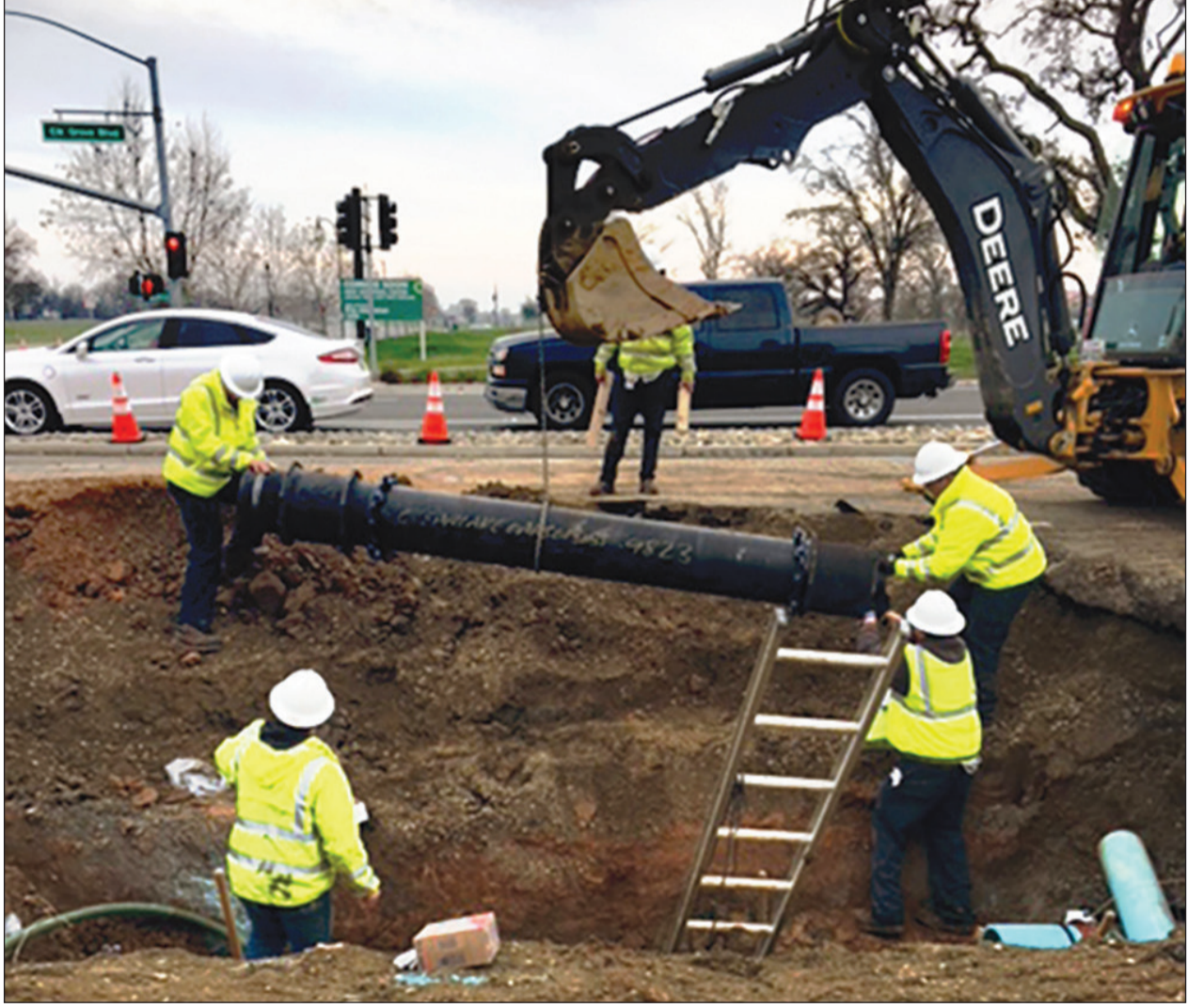
Photo shows Sacramento County Water Agency employees replacing a waterline. Courtesy photo
