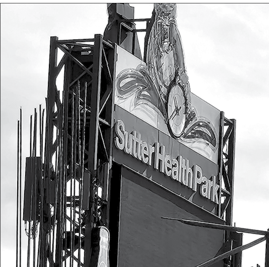
Photo of Sutter Health Park in West Sacramento from October 2024 with construction activities evident.
