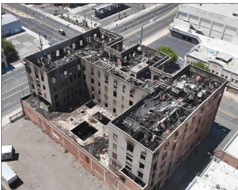
Nearly 6 months after fire destroyed the Hotel Marysville, demolition of its ruins began Wednesday, Dec. 11. Photo courtesy of the City of Marysville
