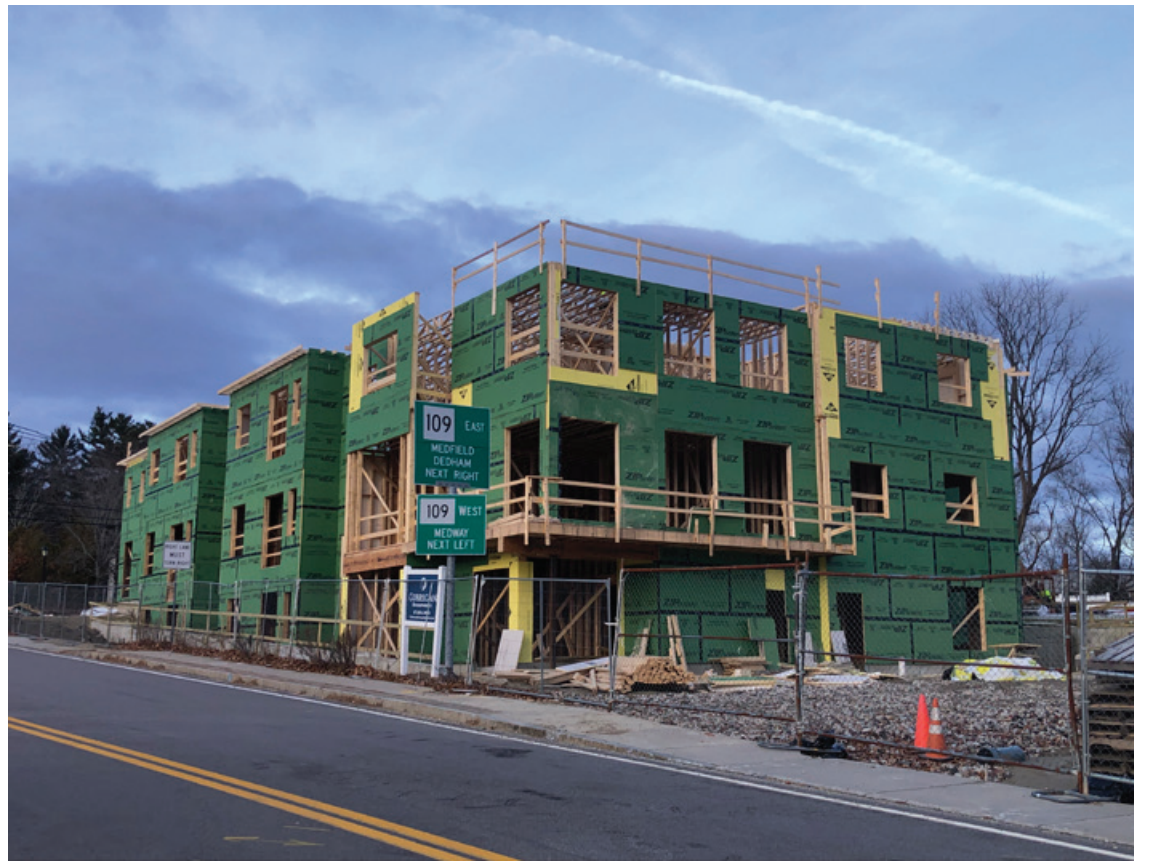
Progress is being made at 1060 Main St. in Millis, at the corner of Main and Pleasant Streets, where a 24-unit apartment building – with six 'affordable' units - is being erected. There will also be one retail space available. Photo credit: Theresa Knapp
