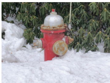
Does your hydrant look like this? The Holliston Fire Department asks residents to "adopt" the hydrant closest to their home and dig it out so it can be accessed in case of emergency. Photo credit: Theresa Knapp
