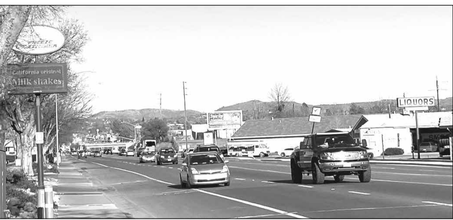
Work will take place at night so as to reduce traffic impacts, which include detours and traffic reduced to a single lane at locations in the westbound direction, between 8 p.m. and 5 a.m. March into June, weather permitting. Photo courtesy of PG&E
