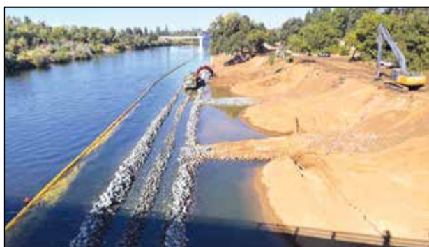
American River Tress members ask that the U.S. Army Corps of Engineers to use different methods to prevent erosion at the American River Parkway. Photo courtesy of American River Trees
