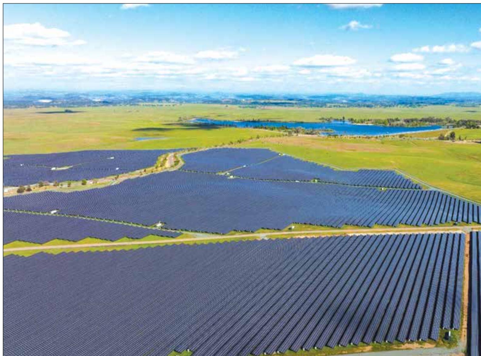
Rancho Seco's energy infrastructure includes a 160-megawatt solar facility, showcasing the Sacramento Municipal Utility District's commitment to clean energy generation. The innovative site combines solar power with sustainable land management through sheep grazing. Photo courtesy of Sacramento Municipal Utility District
