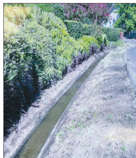
The completed work at the Chesbro Ditch was the first major project overseen by Cory Carskaddon.
