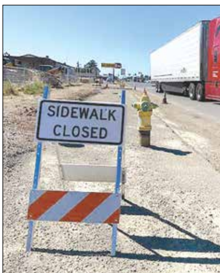
The City of Gridley will move fire hydrants in conflict with Caltrans' construction of a new sidewalk on the northbound side of State Highway 99 as one of two initiatives approved Aug. 18 to improve pedestrian safety.
