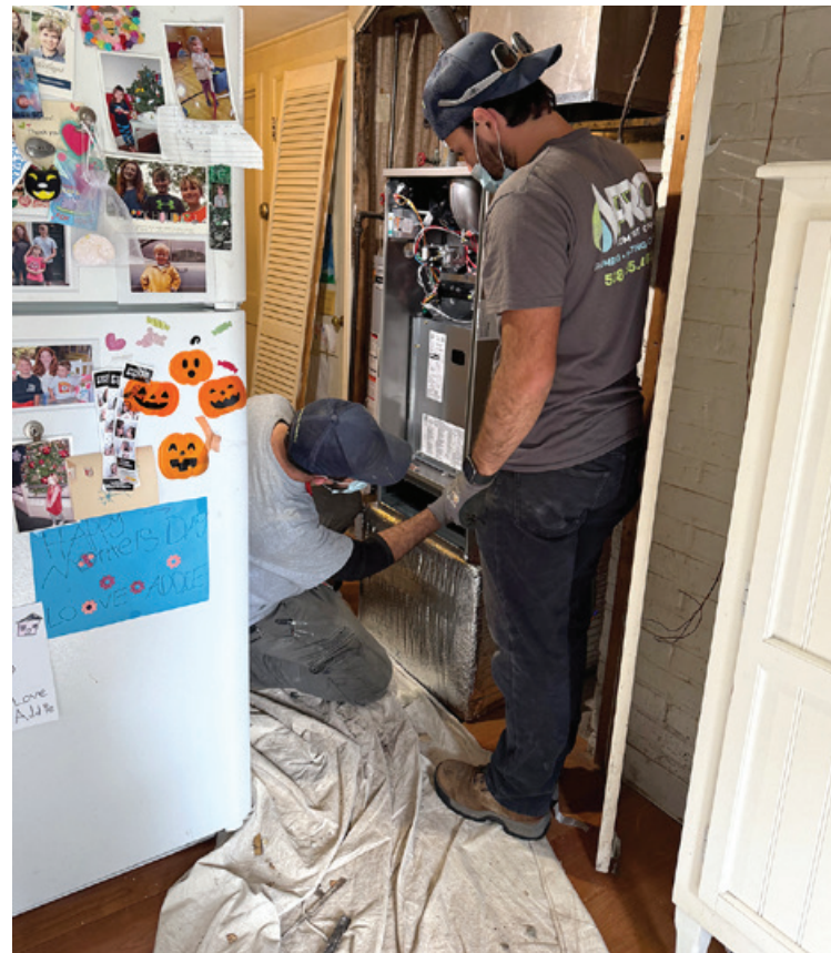
Free furnace installation for the 2024 Natick resident award recipient.
