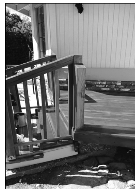
Thanks to the Sacramento County Age-Friendly Community Initiative micro-grant program, repairs such as those to make this deck safe and functional for a Sacramento senior resident were completed. Photo courtesy of Sacramento County
