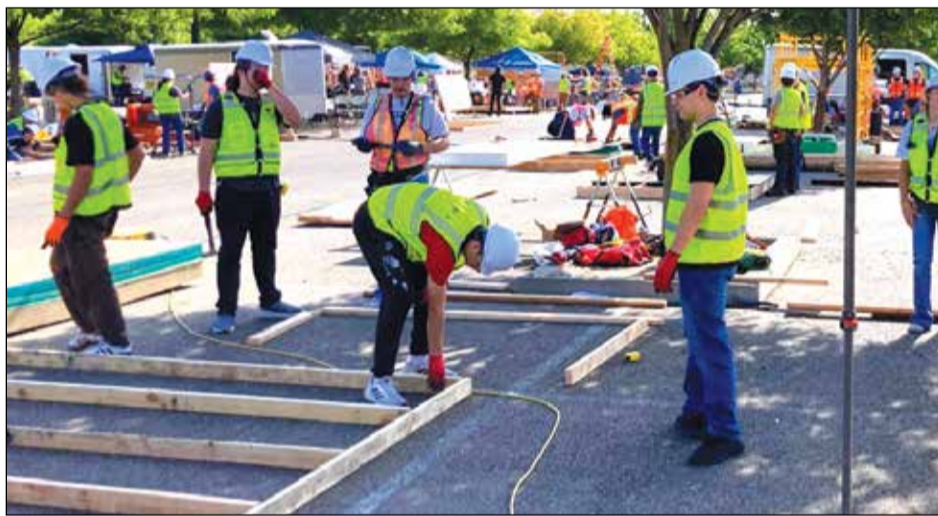
Hosted by the Construction Industry Education Foundation, the 40th annual Design Build Competition brought together high school teams from throughout the region to design and build a structure while meeting strict industry standards. Photo courtesy of San Juan Unified District
