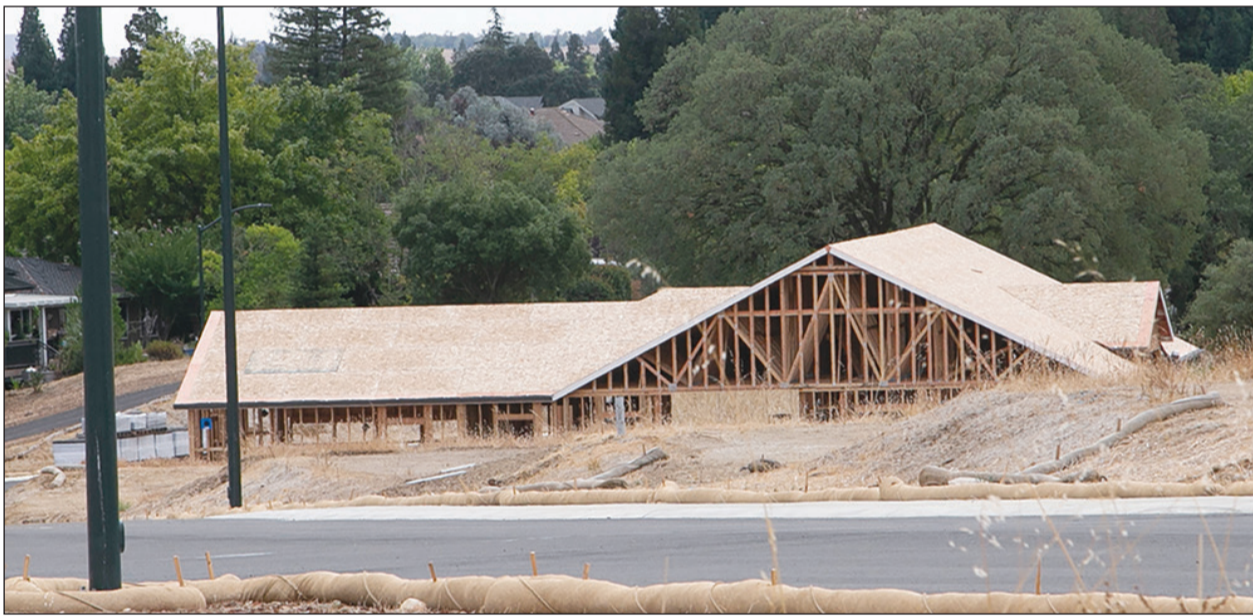
A Terrata Homes model is under construction just inside the Residences subdivision near Escuela Drive. The builder, LGI Homes, spent weeks trying to obtain water meters from the district. Photos by Gail Bullen
