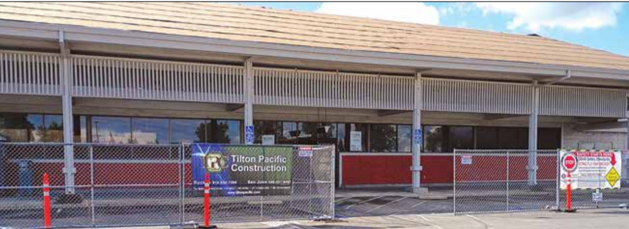
Tilton Pacific Construction, Inc. of Rocklin has begun construction of a new Grocery Outlet store in Sunrise Village. Projected completion is early 2026. Photo by of Thomas J. Sullivan
