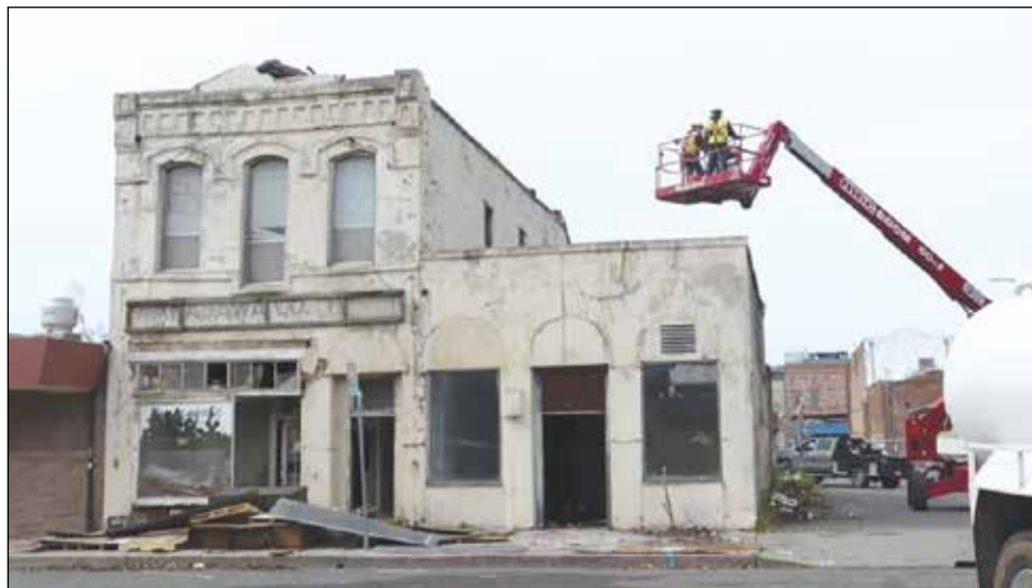
Nakagawa Building and neighboring structure just before demolition. Photo by Chris Pedigo
