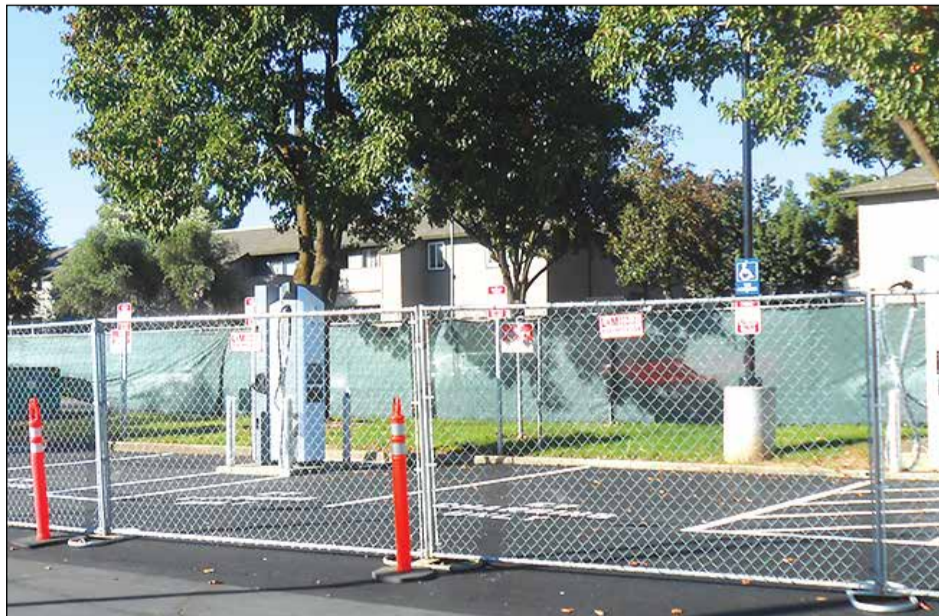
Four new electric vehicle (EV) charging stations have been completed in the far corner of the parking lot at Best Buy in the MarketPlace at Birdcage shopping center and should soon become operational for public use by the end of November. That's according to Kathlynn Carpenter, executive director of the Sunrise MarketPlace (SMP) shopping district. Photo by Thomas J. Sullivan
