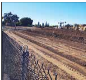
The Carmichael lot is set to be a shopping center development by Pappas Investments, with shop space and drive thru-pads available for lease.
