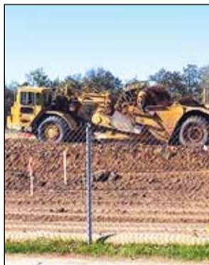
Earth movers can be seen from Manzanita Ave as work begins on Winding Ranch Town Center project. Photos by Paul Scholl
