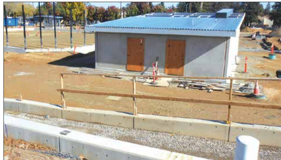
Project work includes the construction of two new tennis courts, a new ticket booth, concession area and upgraded restrooms. Photo by Thomas J. Sullivan
