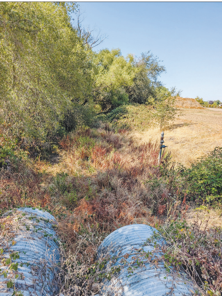
This image shows the condition of the ditch before the clearance work began.
