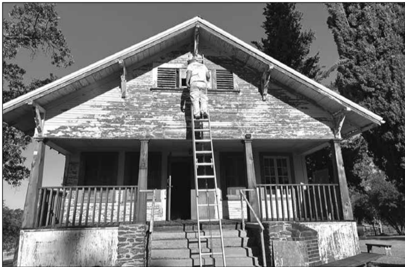
A painter works on stripping and repainting the historic Loma Rica Hall earlier this year, part of the restoration project supported by the Yuba River Endowment and local donors. Photo courtesy of Anita Baker
