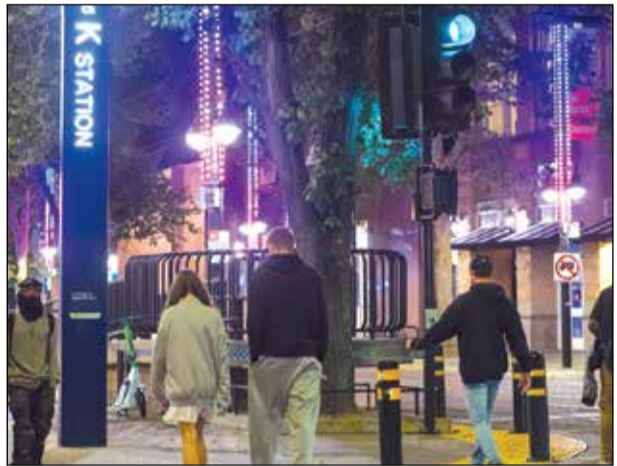
New LED lights have been installed along K Street in Sacramento to promote evening pedestrian activity and safety. Photo by Abbey Wicks
