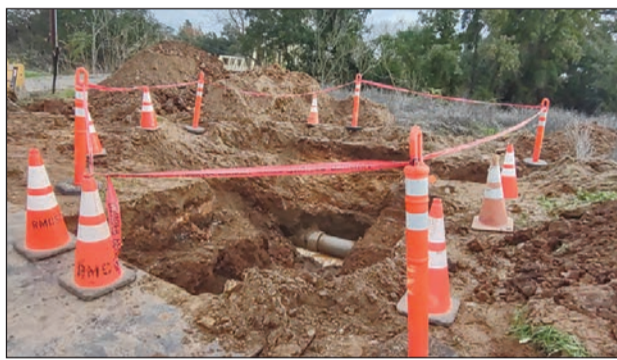
Work is underway to expose a 10-inch pipe that will provide another connection between Lift Station 6B and the 12-inch force main at the Yellow Bridge. Courtesy photo
