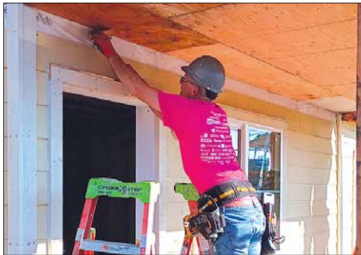
Habitat for Humanity of Greater Sacramento construction crew members said they welcome additional help and encourage skilled and unskilled volunteers to contact Habitat for Humanity of Greater Sacramento to register to work at the job site.
