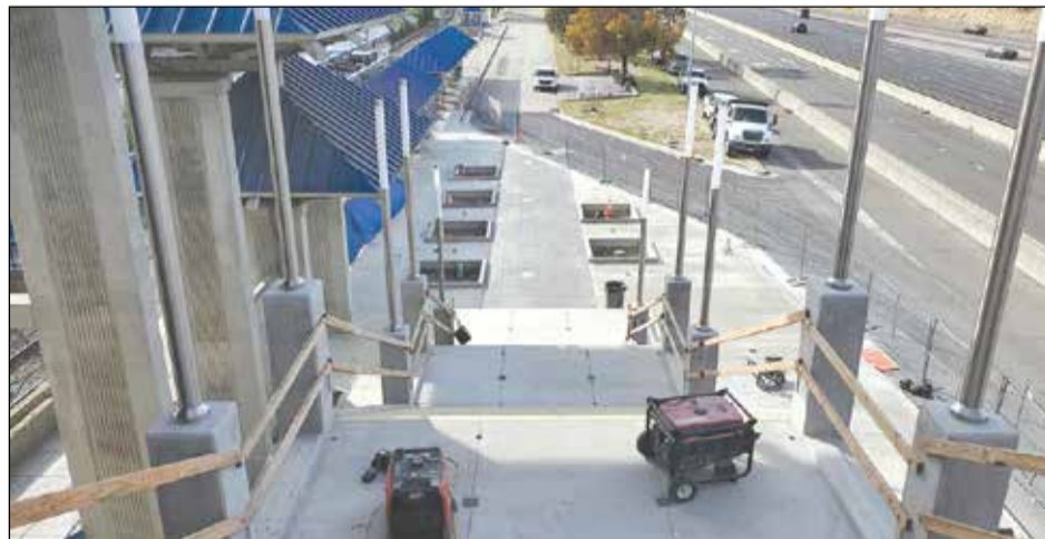
Construction on the Watt/I-80 Transit Center Improvement Project was set to shift to the northbound (east side) of Watt Avenue on Dec. 3, after press time. Photo courtesy of Sacramento Regional Transit (SacRT)
