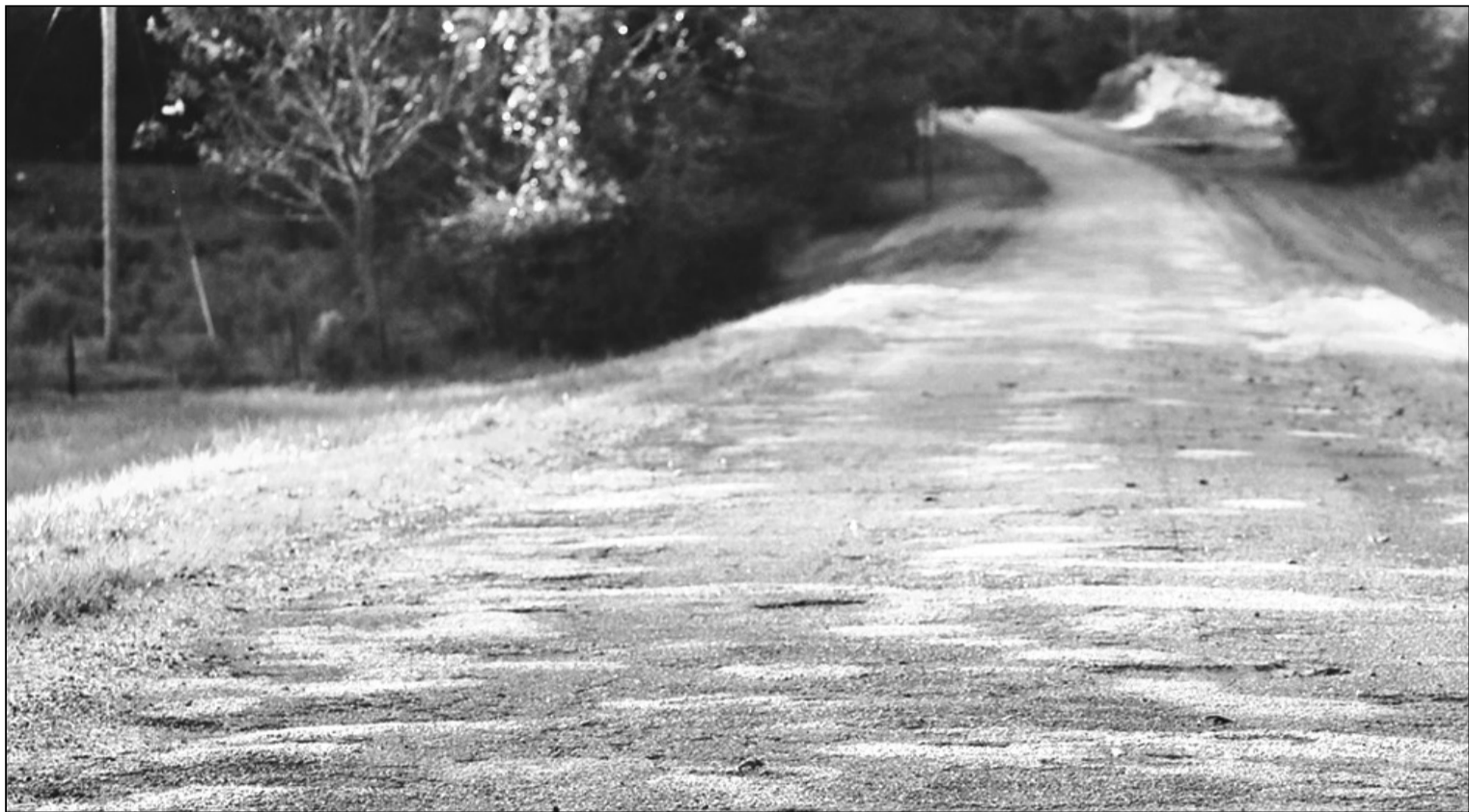
Energy, inland waterways, roads and stormwater received a D. "While California's infrastructure faces significant challenges, this report serves as a clear call to action." Image by Susie Spades from Pixabay
