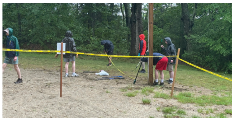
Working in the rain was just one obstacle to renovating Stoddard Park's rundown volleyball court, but Scouts came prepared.
