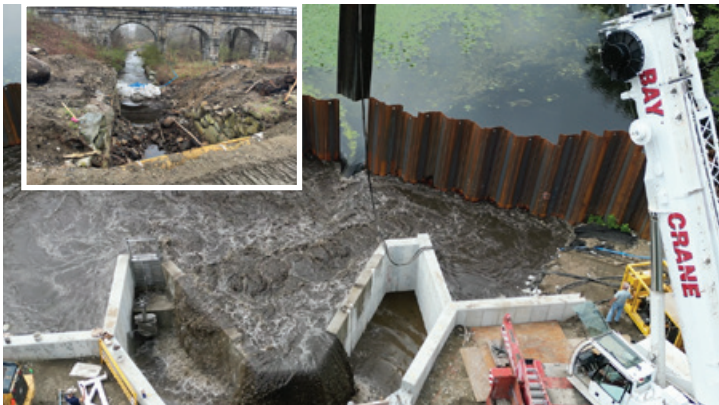
One of Holliston's biggest accomplishments in 2025 was the completion of a 2 ½-year overhaul of the Woodland Street Dam and Bridge. Here, drone footage shows water being released by the temporary dam (shown at inset) once the dam reconstruction was complete. The $3.6 million project cost taxpayers only about $50K.
