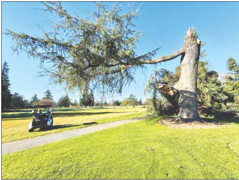
Storm-damaged trees lean over a cart path at Peach Tree Golf and Country Club in Marysville on Dec. 29, following powerful wind gusts that swept through the Yuba-Sutter region on Christmas morning.
