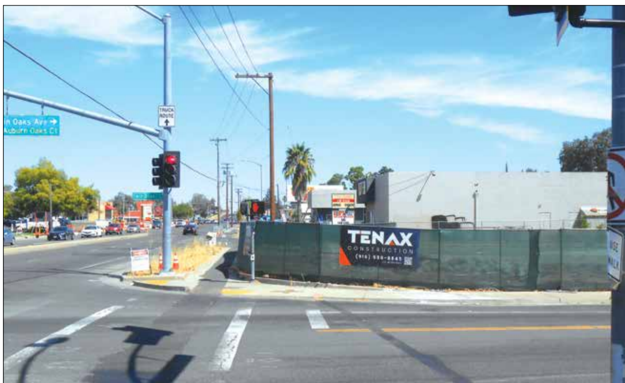
Green fencing surrounds the project site from Twin Oaks Avenue looking north. Photo by Thomas J. Sullivan
