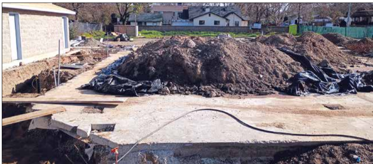
Openings through green construction barrier fencing which surrounds the vacant lot show a new concrete block restroom building now completed and utility trenches dug for pending hookups. Substantial portions of new concrete pads on which food truck vehicles will be parked are visible. Photo by Thomas J. Sullivan
