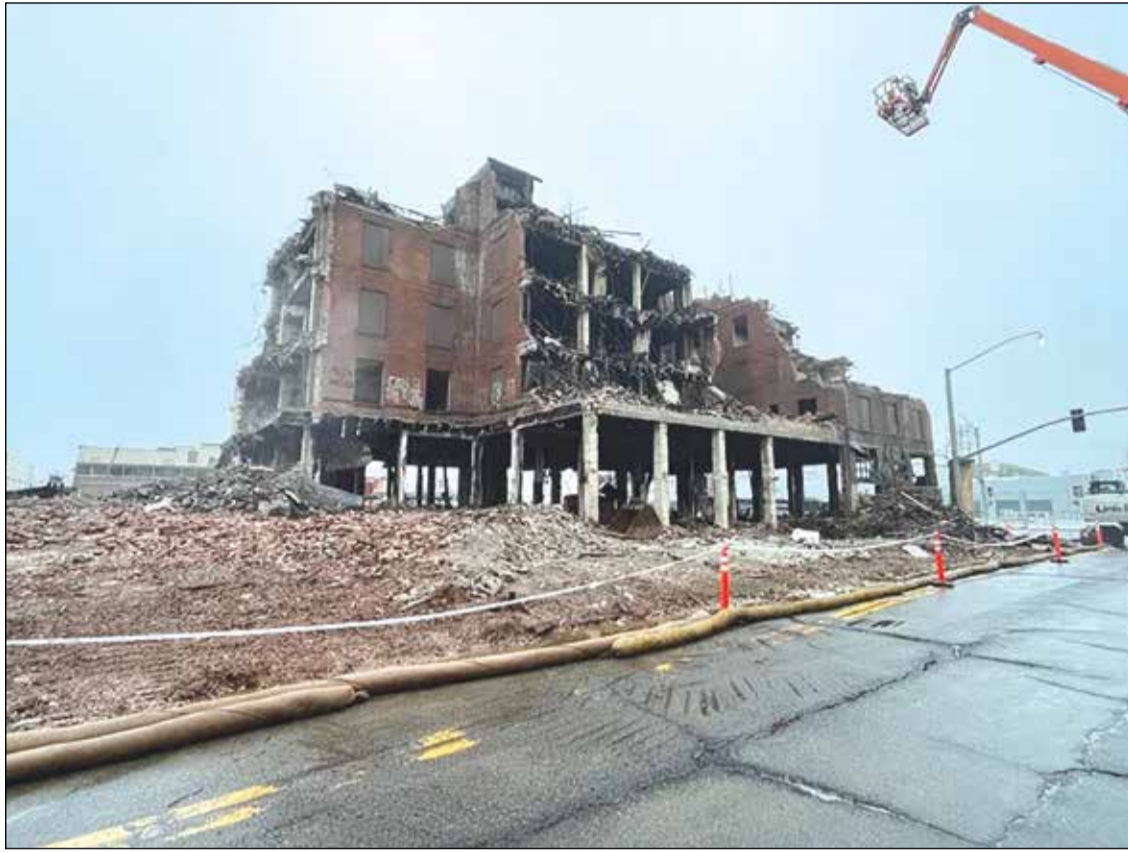
The former site of the historic Hotel Marysville after a June 2024 fire raised significant safety concerns and led to demolition of the building. Built in 1926, the downtown landmark is now the subject of a proposed EPA Brownfields Cleanup Grant application to fund removal of contaminated debris and site remediation. Photo courtesy of Caltrans
