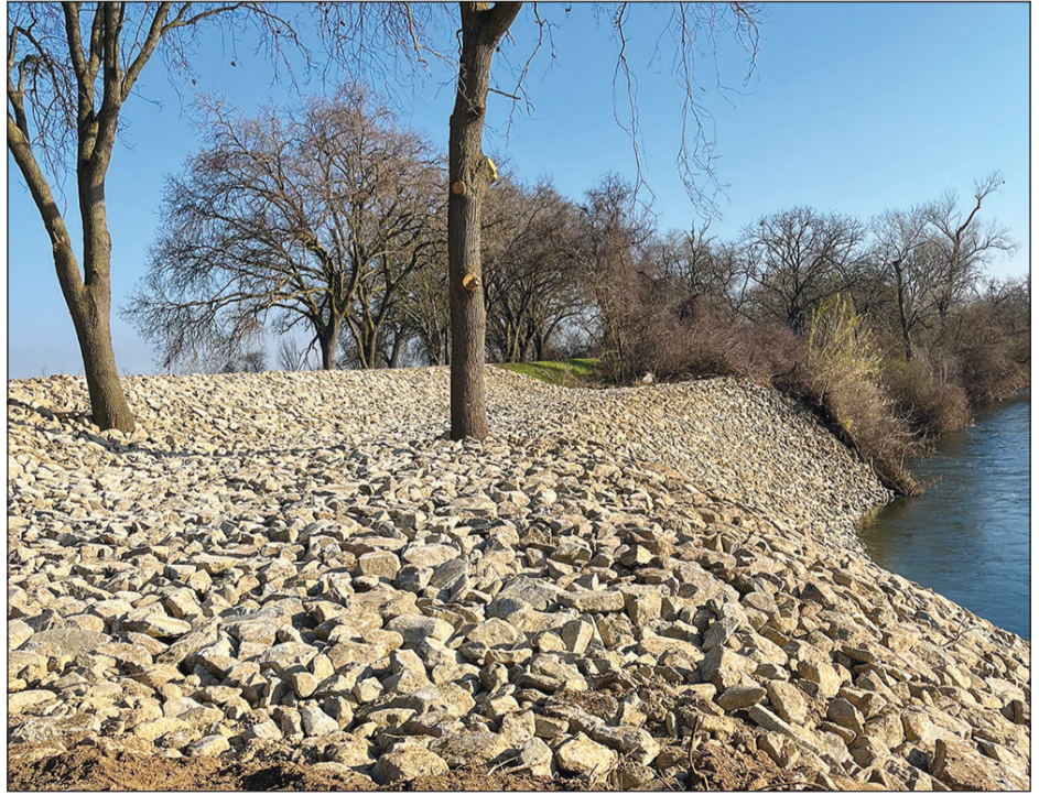
Completed emergency repairs to a levee south of the Folsom South Canal on the Sheldon side of the Cosumnes River are shown after heavy rains in early January. Courtesy photo
