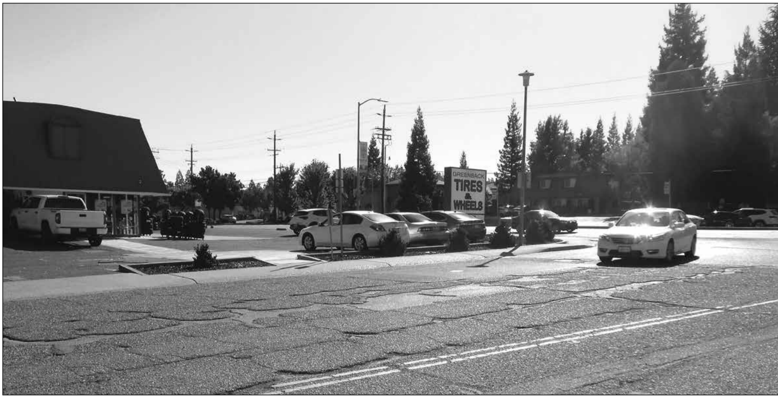
A segment of paving of Sylvan Road from Greenback Lane to San Juan Avenue described by motorists as “rough as a washboard” are included in a comprehensive list of projects scheduled for completion in the 2025 Street Resurfacing Project which is now underway.
