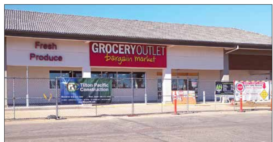
Tilton Pacific Construction, Inc. of Rocklin is finishing construction of a new Grocery Outlet store in Sunrise Village. Photo by Thomas J. Sullivan
