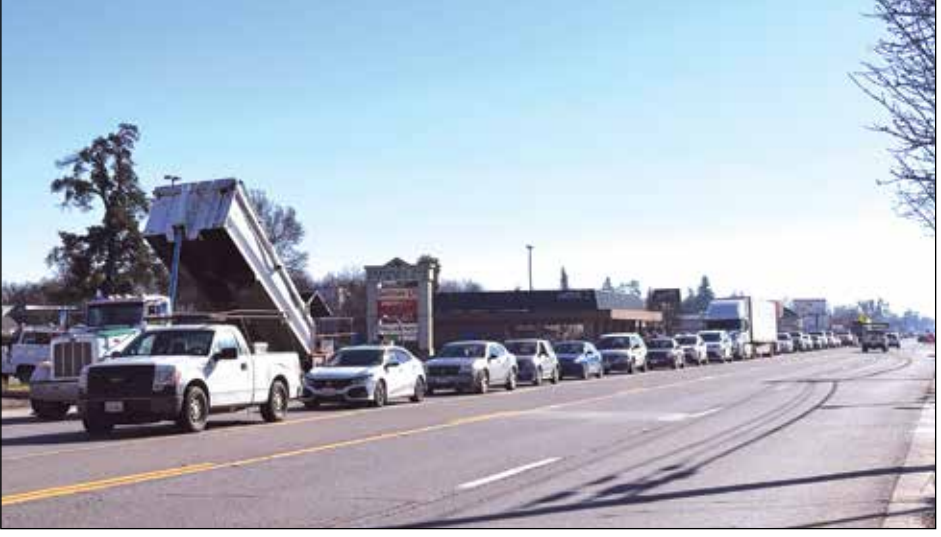
Construction along the Hwy 99 corridor in Gridley backs up traffic as work continues through the business district. Photo by Seti Long
