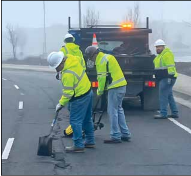
Yuba City Public Works Streets crew complete roadway repairs on Butte House Road on Jan. 26 as part of the city's ongoing efforts to maintain local streets. City officials encourage residents to report road hazards and other concerns through the YC311 service request system. Photos courtesy of City of Yuba City
